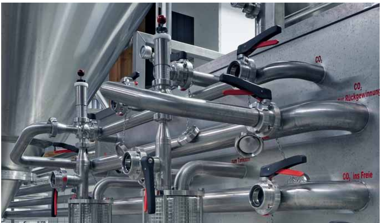
Panel with bunging valves in a brewery
